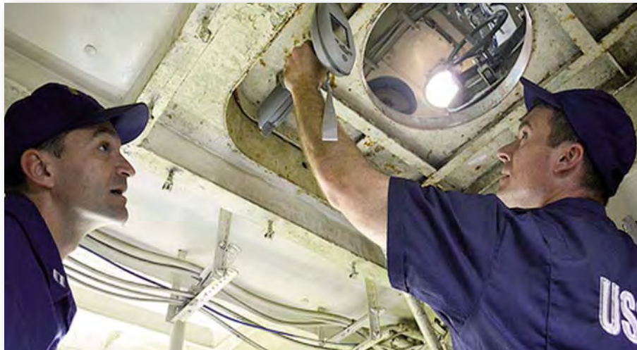
Cooperation between the ship's crew and SEHO auditors are essential. Here the ship's port engineer, LT Igor Landyshev, suggests to LCDR Matt Dooris potential contamination locations. Photo by Auxiliarist Eric Eltinge, HSWL SC (se-fo) Detached San Pedro.
